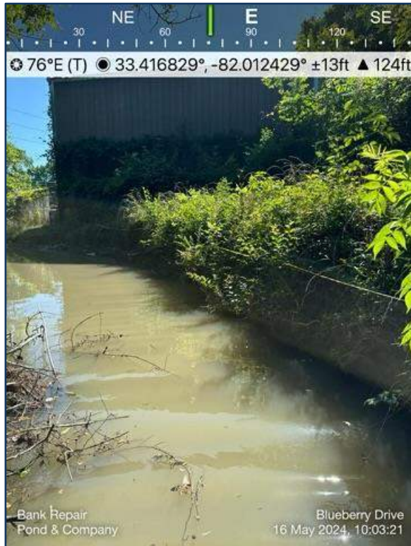
Photograph 5: Looking downstream at right bank; active streambank erosion adjacent to metal building.
