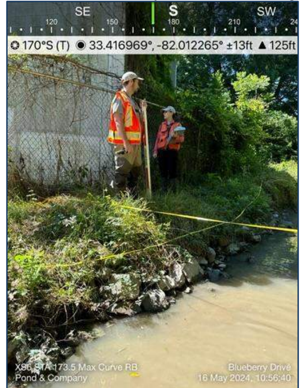
Photograph 8: Looking upstream at right bank; downstream of active erosion adjacent to metal building.
