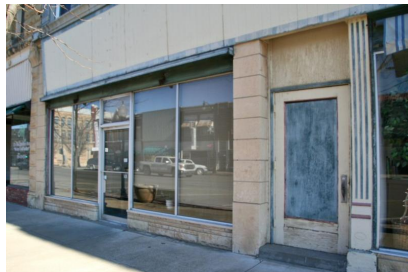
Eagle Block. 312-314 S Summit. Center entrance and north storefront on west facade. 12-11-2017. B. Spencer
