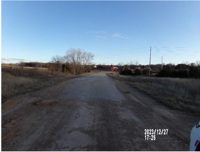
End of pavement approx 400 feet north of intersection, south of site taken 12/27/2023 by Josh White
