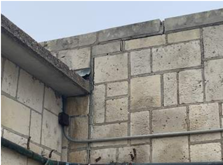
Damage due to settlement in the opposite (northeast) corner of the building from the previous photograph.
