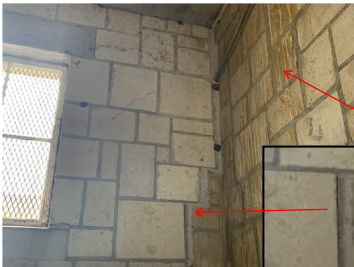
Note a gap has opened up since the tuck point repair indicating continued movement in the structure. This is in the storage room on southwest corner of building.
