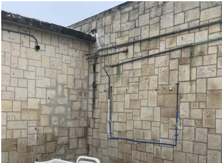
The next two photos show earlier tuck point repairs in the masonry joints to address cracking due to settlement.
