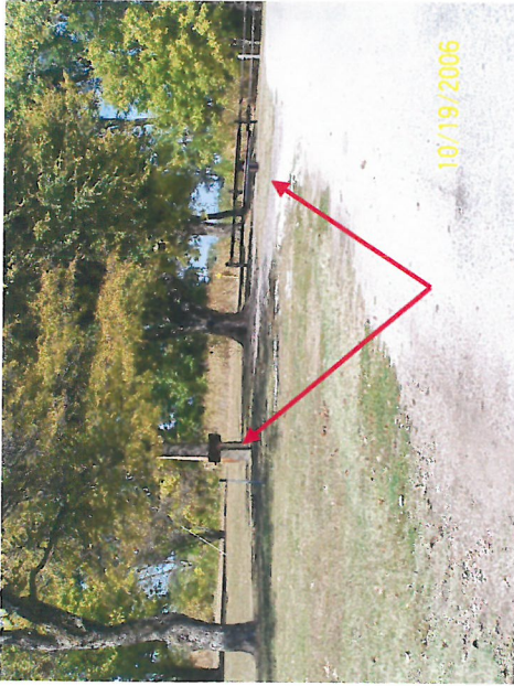
Amenities such as fixed picnic tables and BBQ grills are not on accessible routes.
