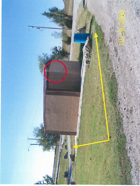
The restrooms are not on an accessible route. Signage is located off the route to the entrance.
