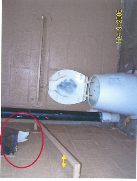
Restrooms have toilet paper dispensers mounted above side grab bars and 3" between bars and wall (yellow arrow).
