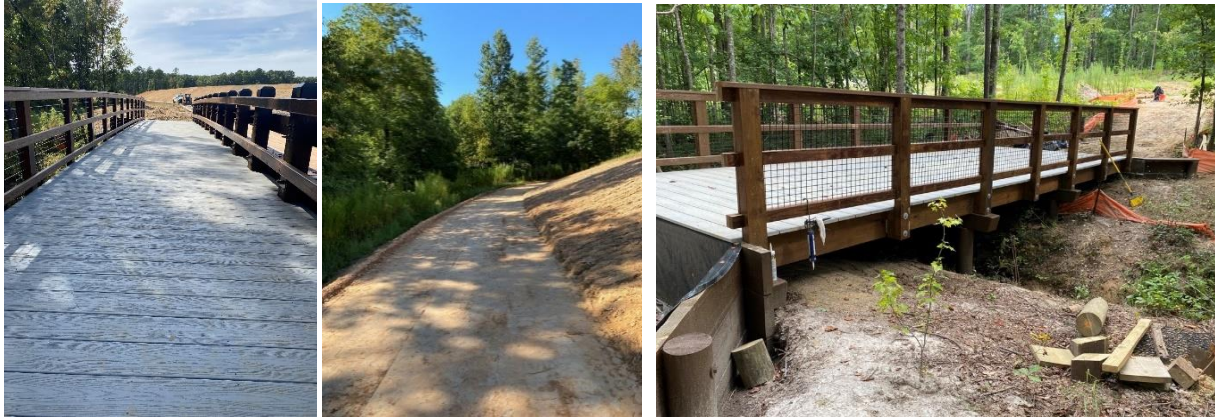
FIGURE 10/11/12: PEDESTRIAN BRIDGES AND BOARDWALKS ALONG CROSS COUNTRY TRAIL FOR PLEASANT PARK IN THE TOWN OF APEX
