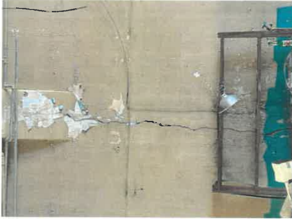
W Wall 206 daylight seen through cracks
