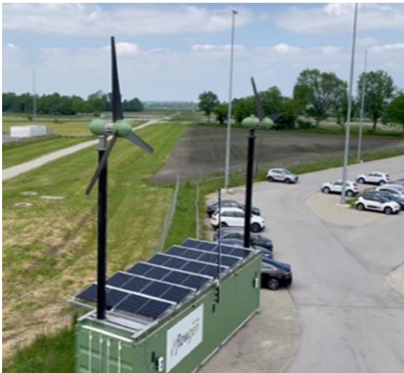
FIGURE 18: 10-KW MICROWIND TURBINES WITH SOLAR AND BUILT-IN BACKUP ENERGY STORAGE. SOURCE: FLOWGEN
