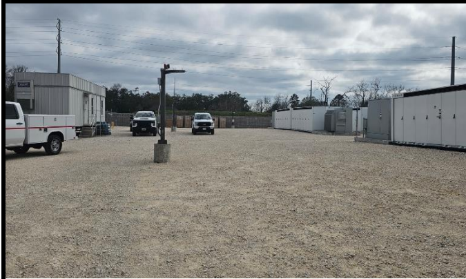
View onsite of battery units
