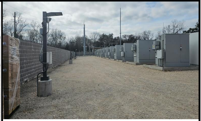
View onsite of battery units
