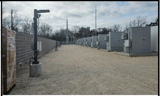
View onsite of battery units
