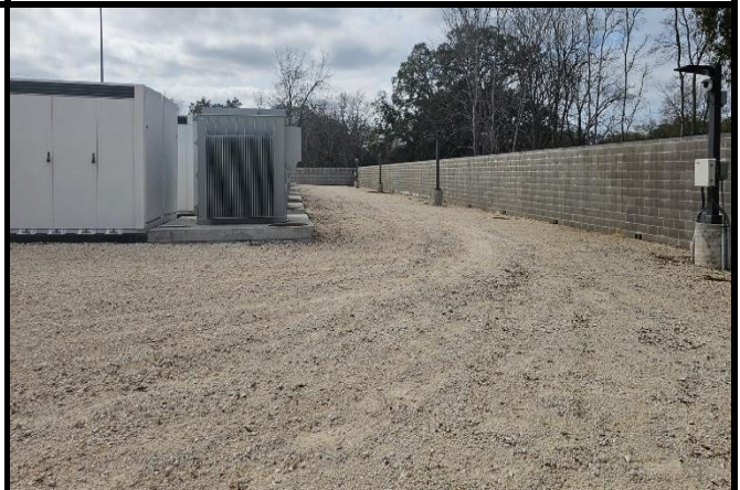
View looking on site of Battery Units and access drive
