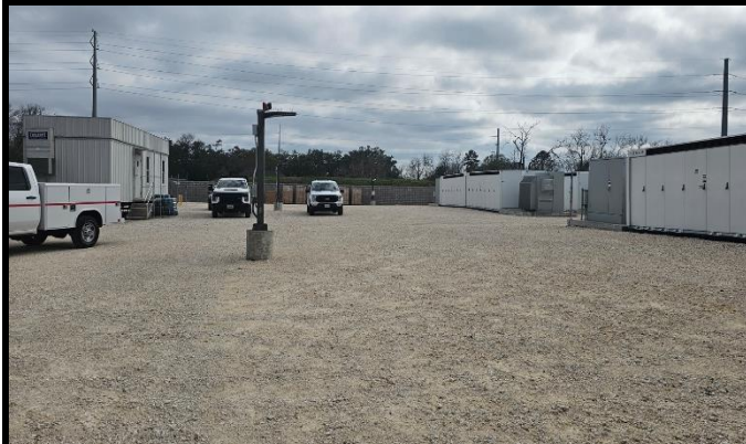
View onsite of battery units
