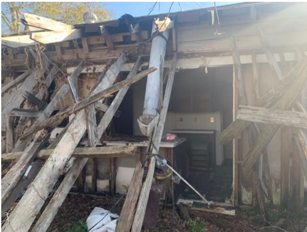
Kitchen visible - back wall missing
