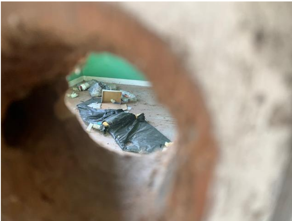
Doorknob hole in front door - Evidence of vagrants occupying unsafe structure
