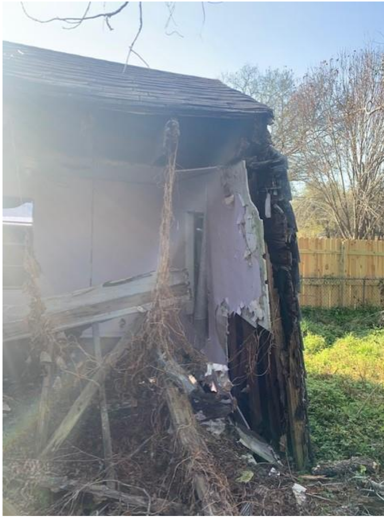
Back bedroom collapsed
