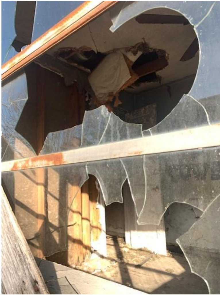
Broken windows, ceiling caved in
