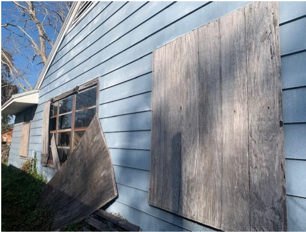
Windows boarded, windows broken, structure leaning
